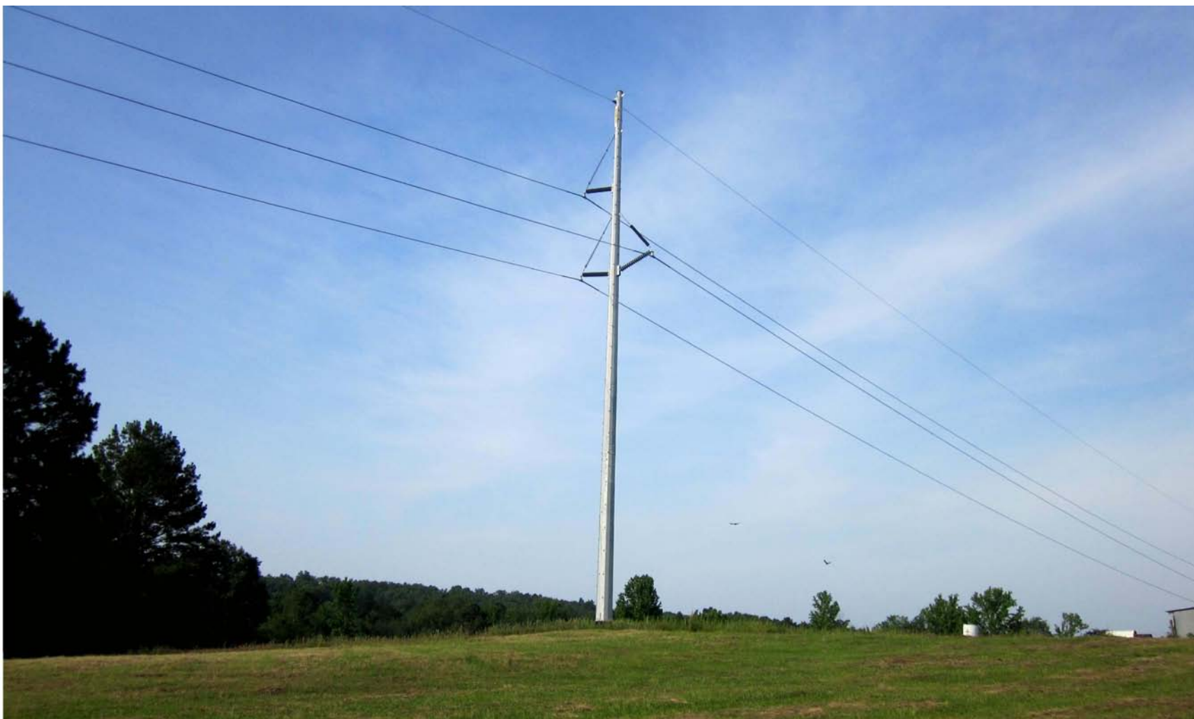
Figure 2. Typical T-Line Pole Configuration.
